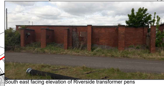
1. Redundant transformer pens
